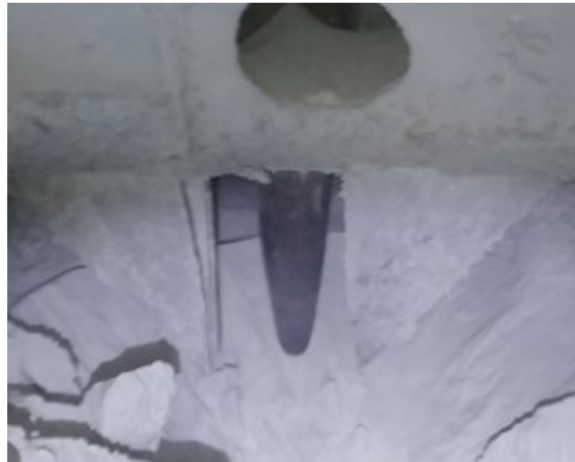
Figure 1. Crust breaker in aluminium reduction cell.
